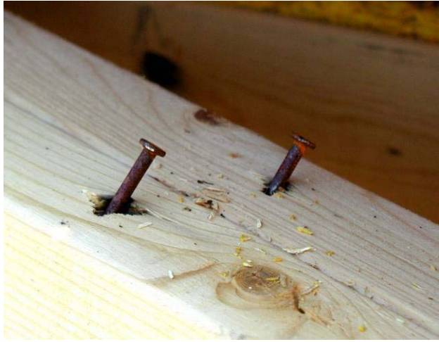
Nails in the double top plate of the specimen T4-2 (sheathing is pulled away to expose the nails)
